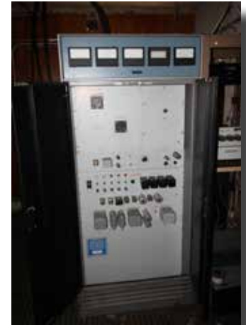
The former WABY CCA 1000-D transmitter
