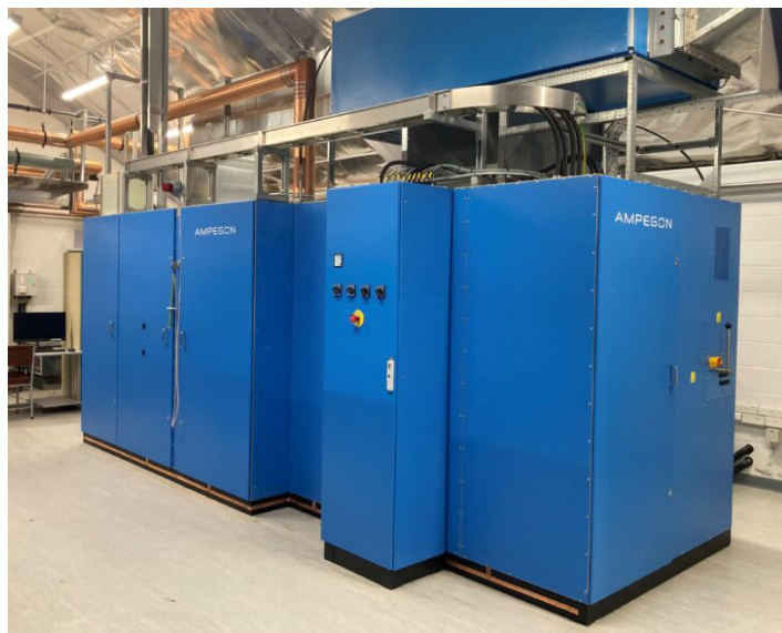
RNZ's new 100 KW Ampegon shortwave transmitter system
