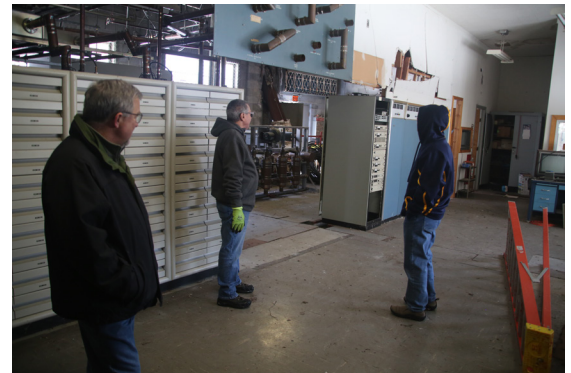
WTEN Chief Engineer Steve Pingelski (left) looks on as club members survey the station's former analog transmitter building in the Helderberg Mountains.
