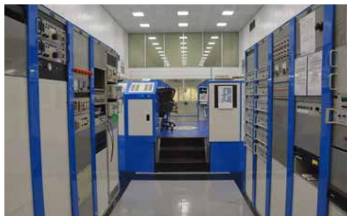
The Control Room in the U.S. government's Edward R. Murrow Transmitting Station near Greenville, North Carolina.
