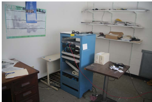
Space for the repeater is located in the former WTEN engineering office at the station's old analog transmitter site. EGARA also installed a wi-fi "hotspot" and security cameras to monitor the site.
