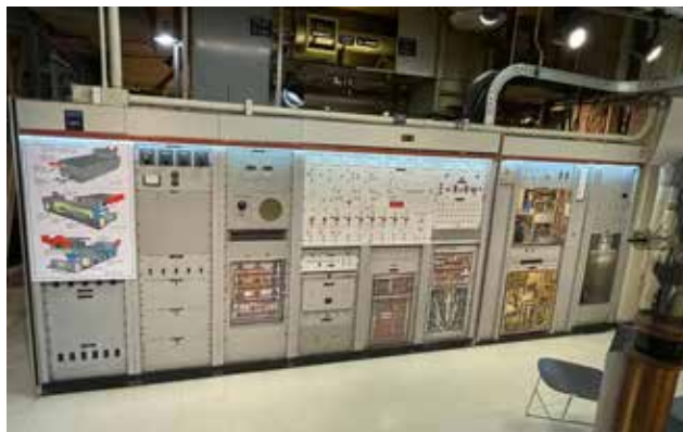
One of the massive VOA transmitters on display. At its peak the facility had six transmitters broadcasting with 250 kW and two transmitting with 50 kW.
